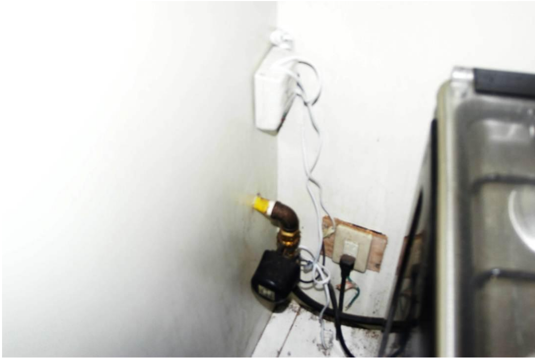
Figure 48 – gas detector, shut-off valve and power supply in Unit 303B Note double socket outlet on end wall, only range plugged in
